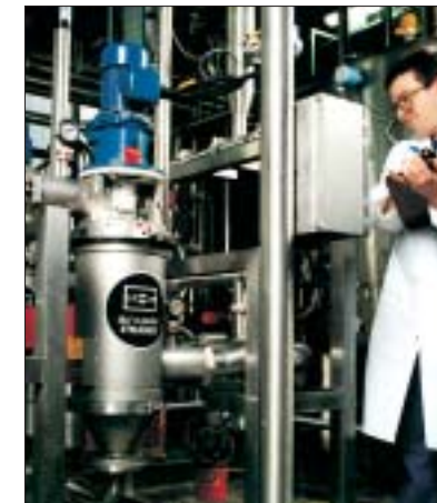
Russell Eco Self-Cleaning Filters® provide pre-filtration at a factory of H.P. Bulmer - Cider manufacturers
